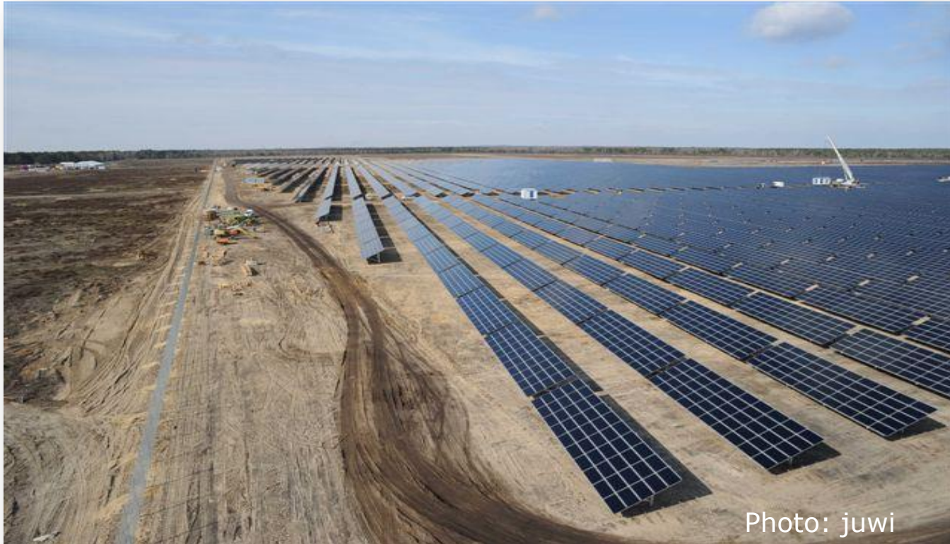
Germany, Lieberose, 53 MW Due Dilligence, Construction Supervision, Inspections
